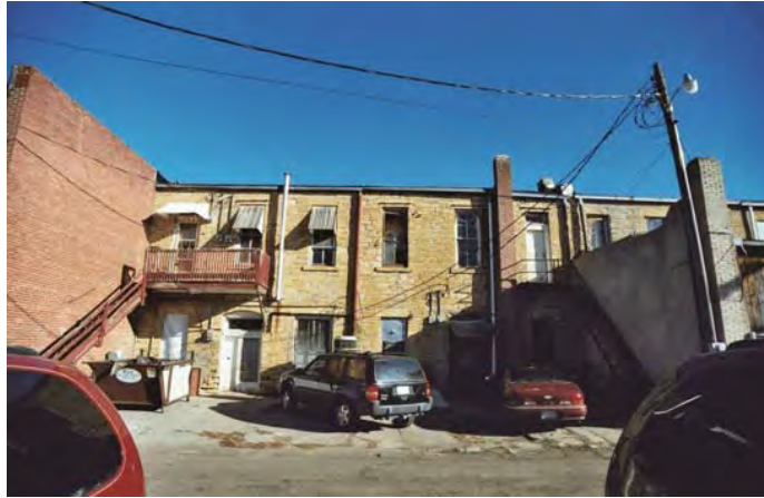
Photo 8: A rear facade open to parking which does not exhibit a well maintained attractive appearance.
