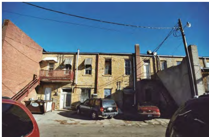
Photo 8: A rear facade open to parking which does not exhibit a well maintained attractive appearance.
