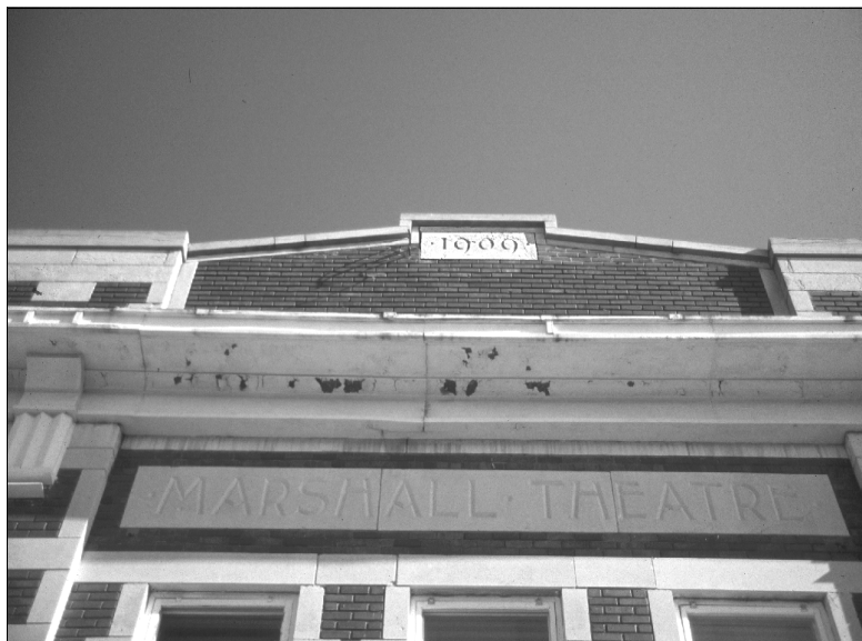
Photo 4: Example of brick and stone cornice. Note metal soffit material requiring maintenance.
