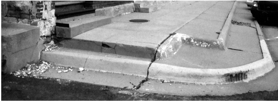
Photo 3: Deteriorated and awkward steps and curb conditions contribute to tripping hazards and limit ease of access to businesses along Main Street.
