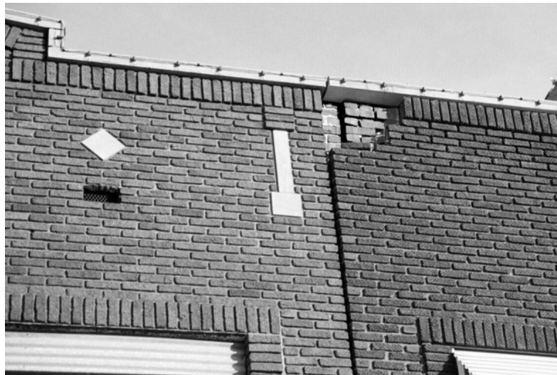
Photo 3: Building cornice exhibiting parapet damage that leads to moisture penetration into the wall system contributing to structural deterioration.
