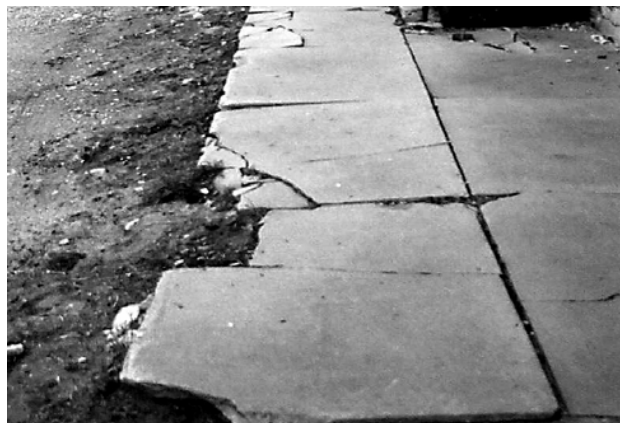
Photo 2: Deteriorated sidewalks contribute to hazardous walking conditions and negatively impact the character of downtown areas.
