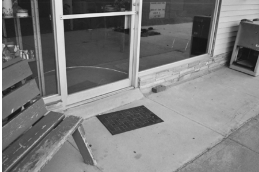
Photo 1: Example of improper “ramp” modification at building entry that still limits access.
