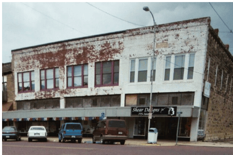
Photo 2: A building facade needing maintenance and paint removal/cleaning and repainting.
