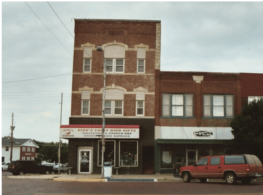
Photo 2: View of building exhibiting vertical orientation. Note inappropriate infill and undersized replacement windows.
